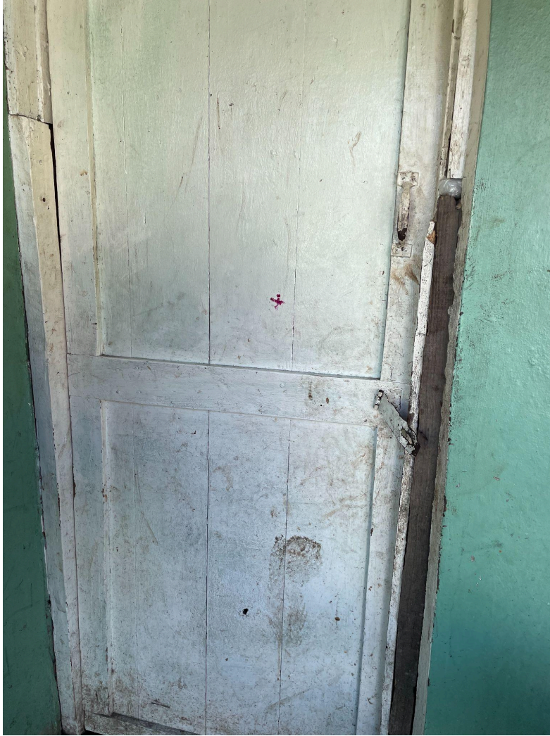
Broken latch along with boot print and scuff marks from repeatedly kicking the door / Pestillo roto junto con huellas de botas y marcas de desgaste por patear repetidamente la puerta
